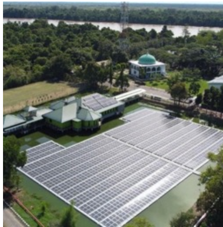
Floating solar PV 467 kWp at CPBL | Floating solar PV 467 kWp di CPBL
